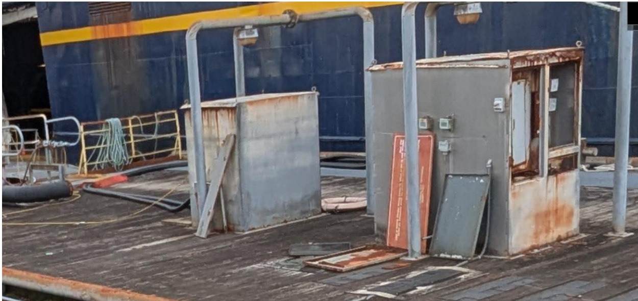
Figure 7- Berth 2 Existing Shore Power Boxes, Observed October 2025
